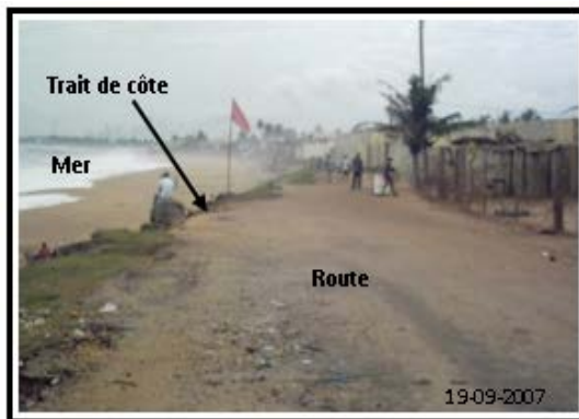
Figure 6. Road interrupted by erosion at Port-Bouët lighthouse.
