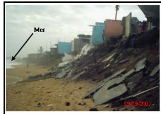
Figure 7. Damages caused by Aug. 2007 storm at the west side of the lighthouse.
