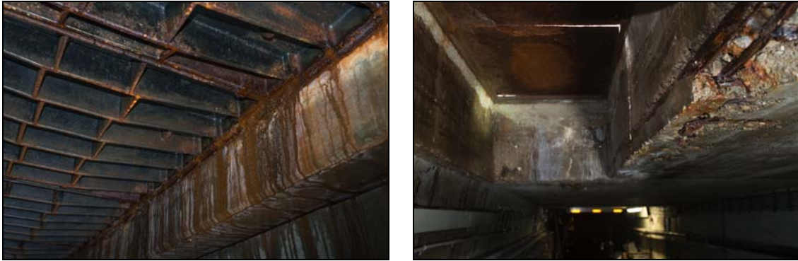
Figure 2. Leaky hatch cover - left damage class 2 – water seepage and corrosion at the steel cover; right damage class 4 – reinforcement corrosion with reduction of cross section and concrete spalling.
